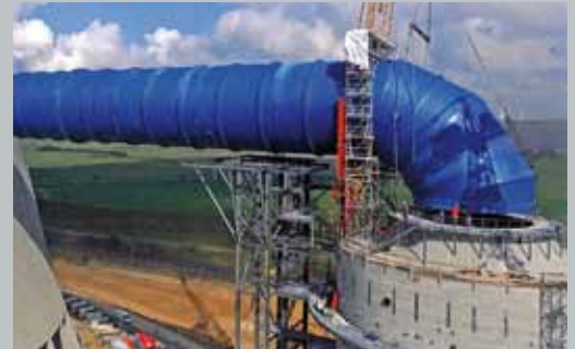
Flue Gas Duct in a Power Plant in Germany
