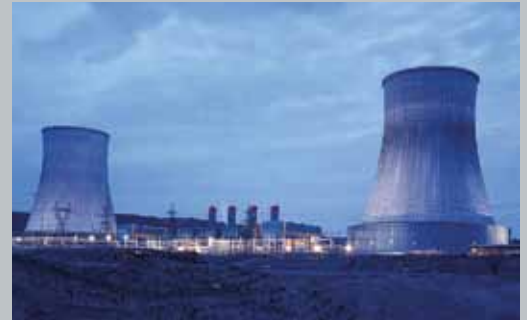
Heller Indirect Dry Cooling Systems in a Power Plant in Turkey
