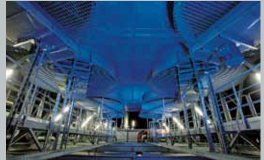
Air Fin Cooler - Combined Cycle Power Plant in Münster/Germany
