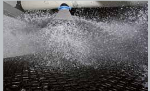
Water distribution in a cooling tower
